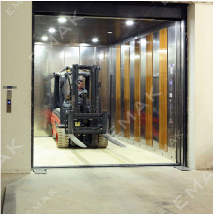
Kare Warehouse - Showroom / ANKARA EMMAK Hydraulic Cargo Elevator Rated Load: 7 Tons
